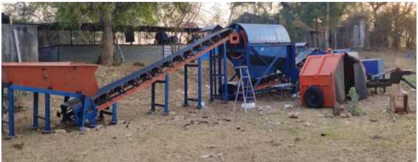
Biomass management plant
